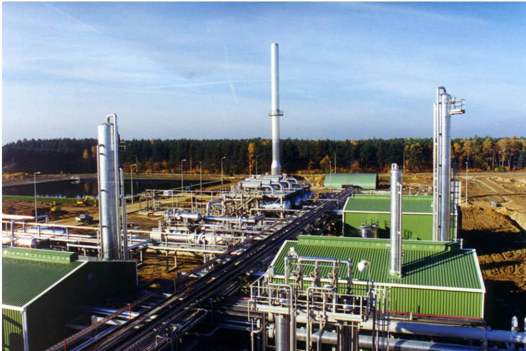
Polish Oil and Gas Company – Dębno, Poland
