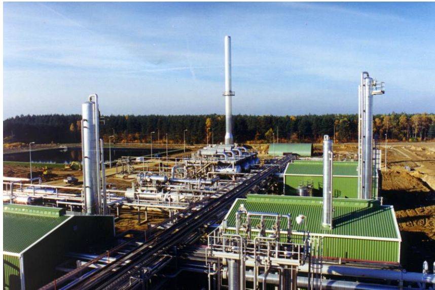
Polish Oil and Gas Company – Dębno, Poland
