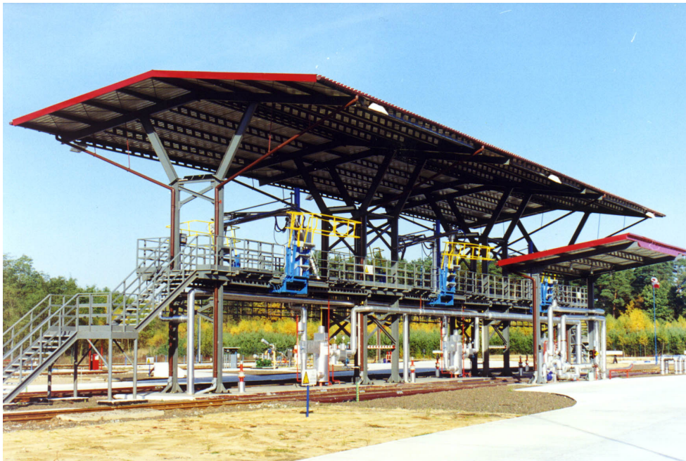
Polish Oil and gas Company – Dębno, Poland
